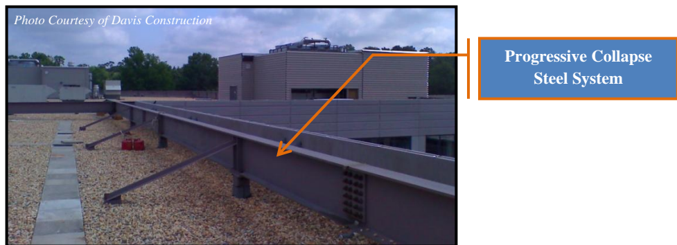
Figure 2 | Progressive Collapse System Installed
